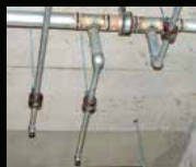
Fire Sprinkler Systems
