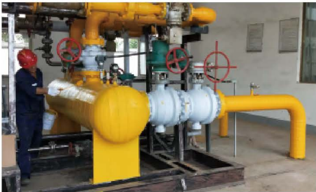
Gas Station Corrosion Prevention In China Resources
