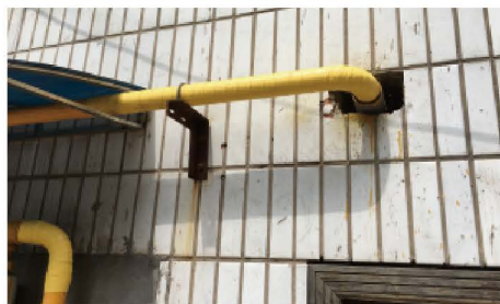
Corrosion prevention for through-wall/floor pipeline
