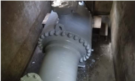
Valve Chamber Application Beijing Gas(Before Corrosion Prevention)
