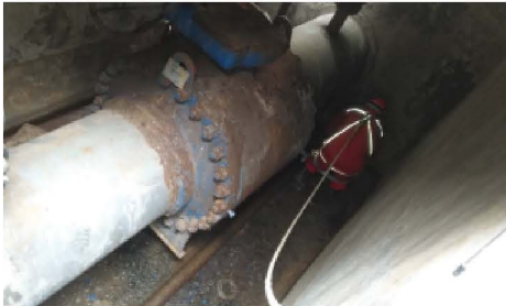
Valve Chamber Application Beijing Gas(Before Corrosion Prevention)
